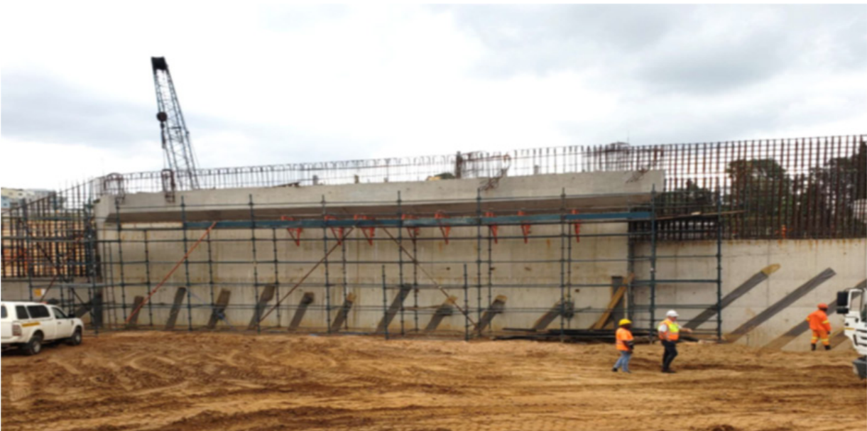
Upgrading of K73 between Woodmead Drive and Allandale Road (D58) Mushroom farm.
