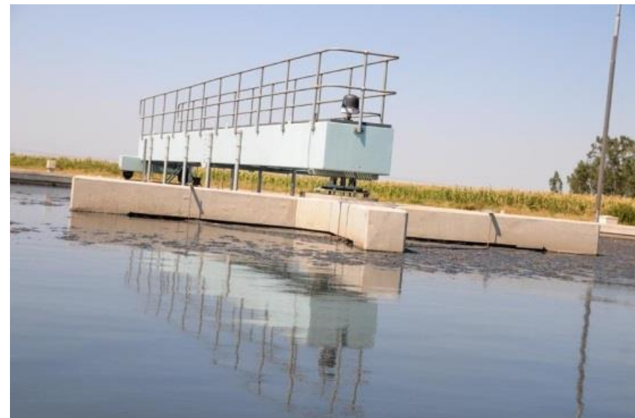
Part of the wastewater treatment works.
