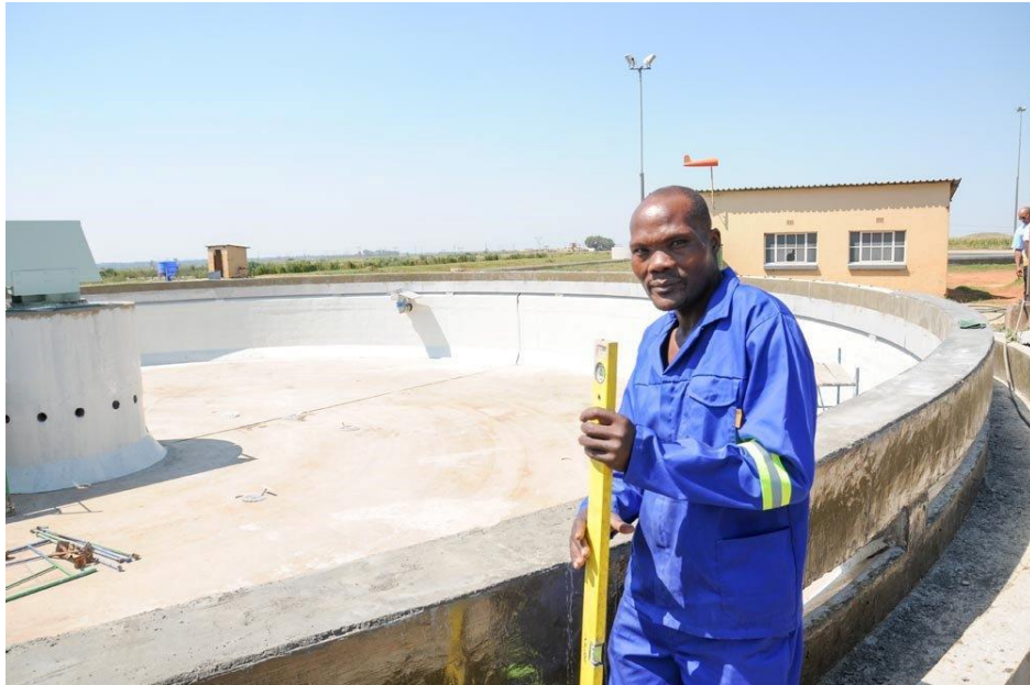
The wastewater treatment works project will assist future human settlement projects, as the previous reservoir did not have enough capacity to accommodate the increase in residential areas.
